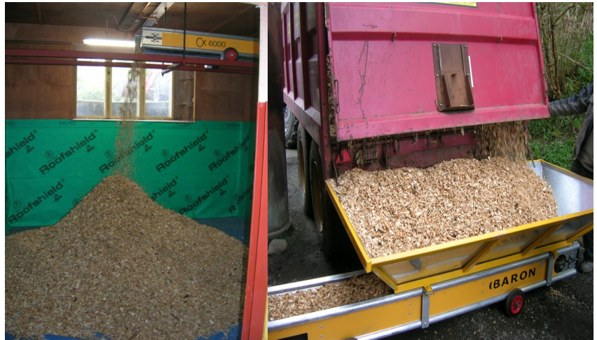
Customers woodchip, being delivered into the fuel store
