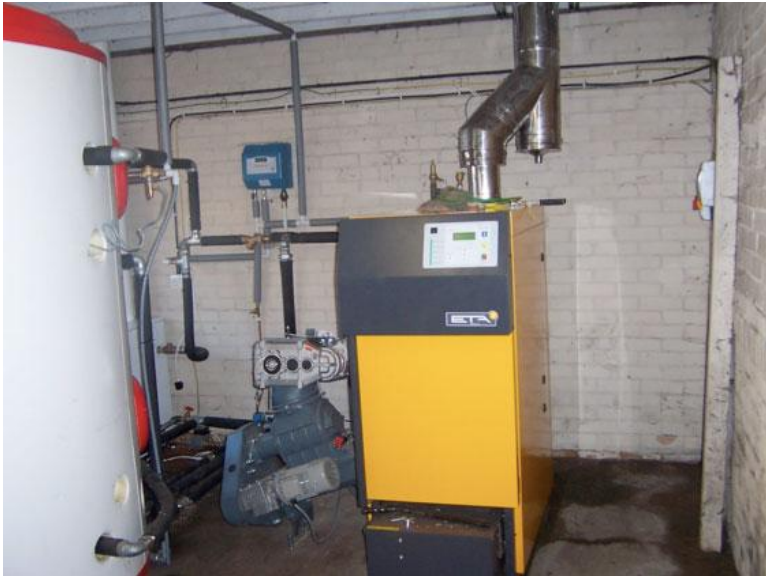
Completed installation of the ETA HACK 50KW Woodchip, biomass boiler. A 50KW oil boiler can be seen in the background, this will be used as a back-up if the boiler runs out
