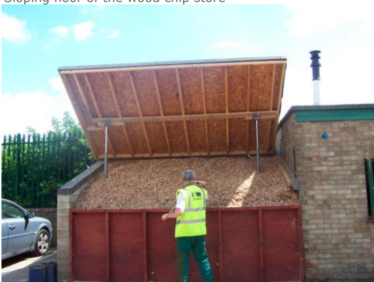
Completed and filled wood chip store
